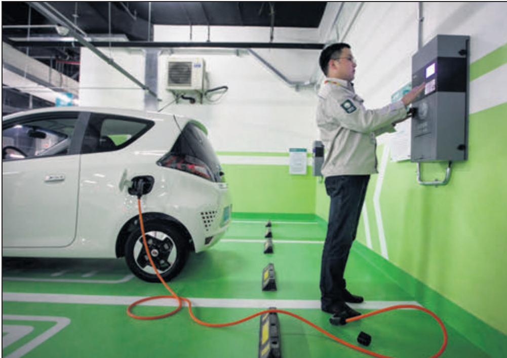
A technician from State Grid Shanghai Municipal Electric Power Co inspects the charging piles, or power ports, in a parking lot before they are put into operation. XINHUA
